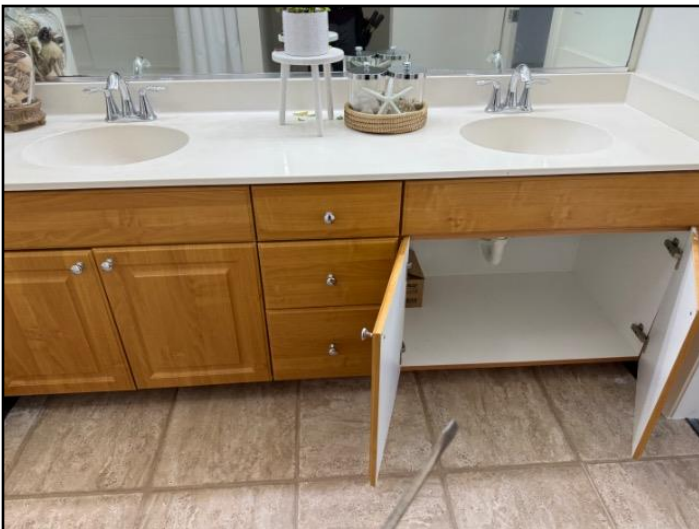
Leak @right side vanity sink
