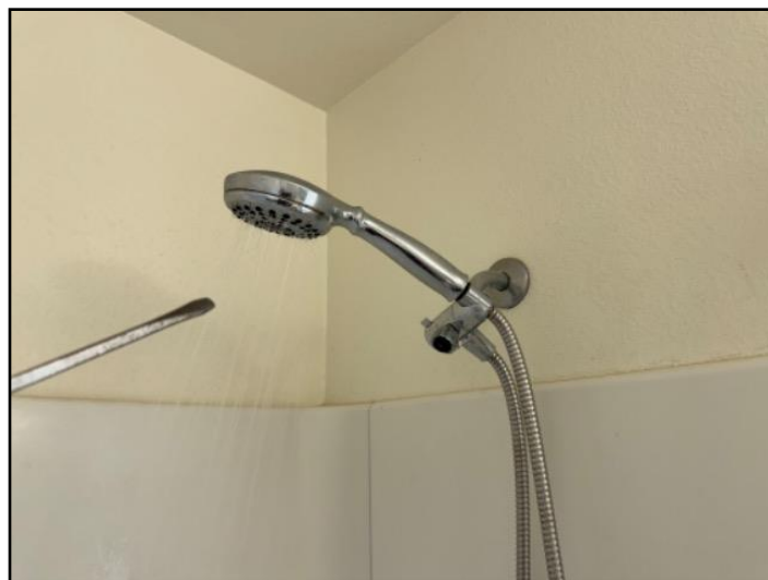
Shower head damaged
