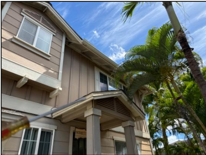
Trees or shrubs too close to building
