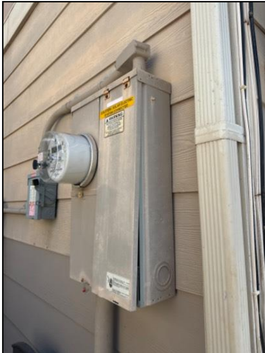
Breakers - exterior wall
