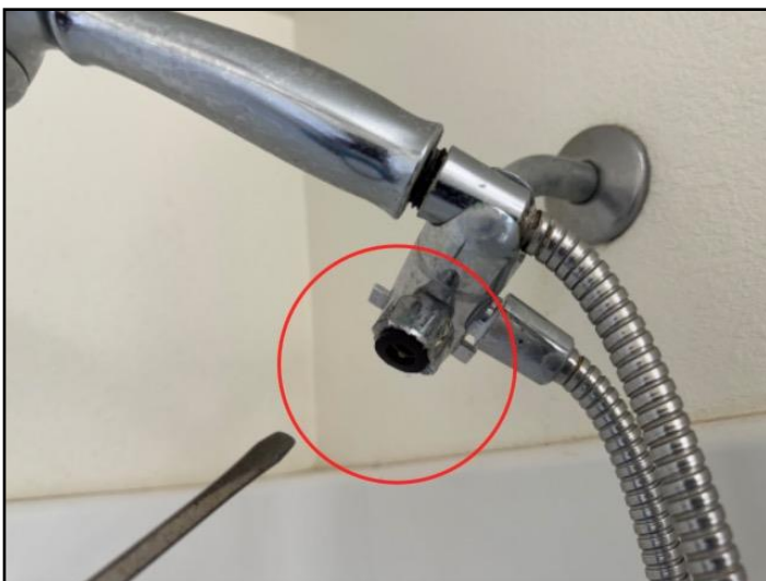
Shower head damaged
