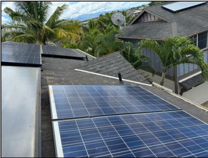
Solar panel array
