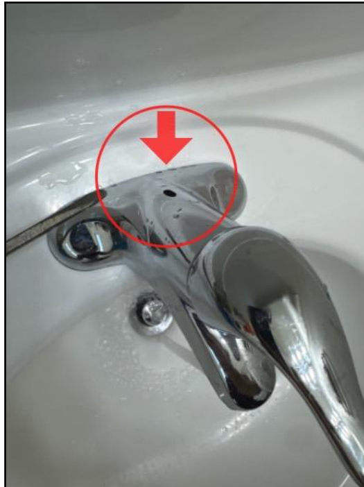
Drain stop missing
