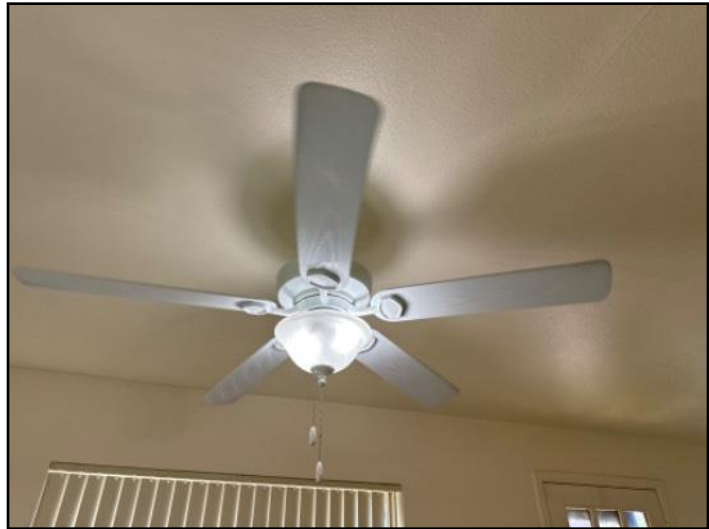
Ceiling Fans tested functional
