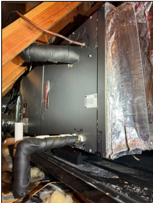
Attic air handler
