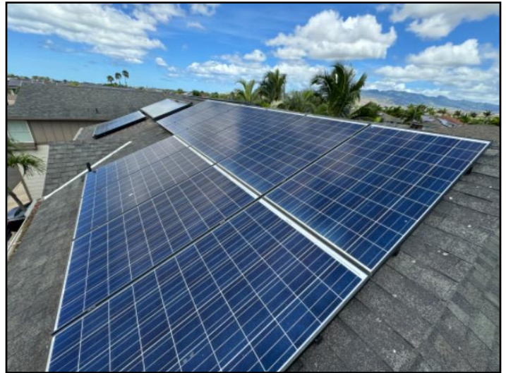
Solar panel array
