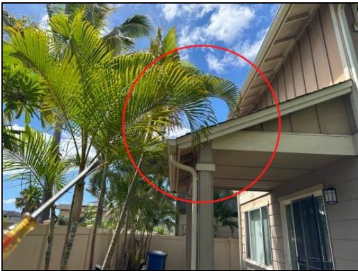
Trees or shrubs too close to building
