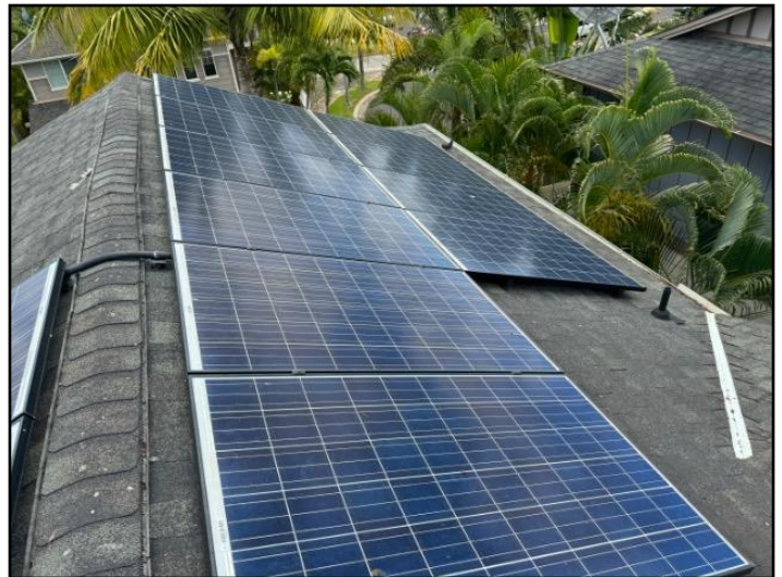
Solar panel array
