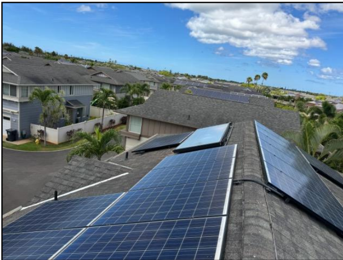
Solar panel array
