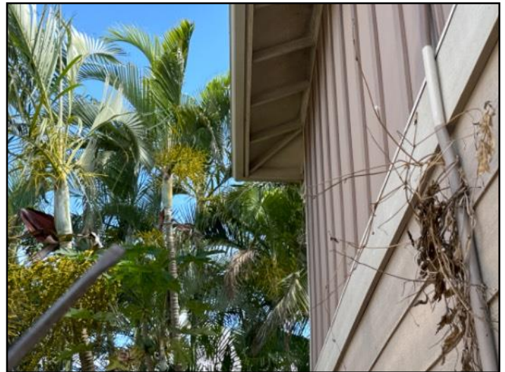
Trees or shrubs too close to building
