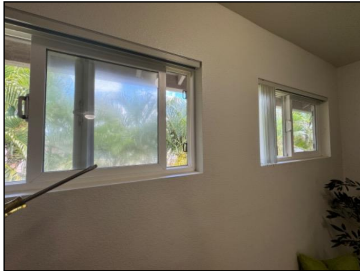
Lost seal on double glazing
