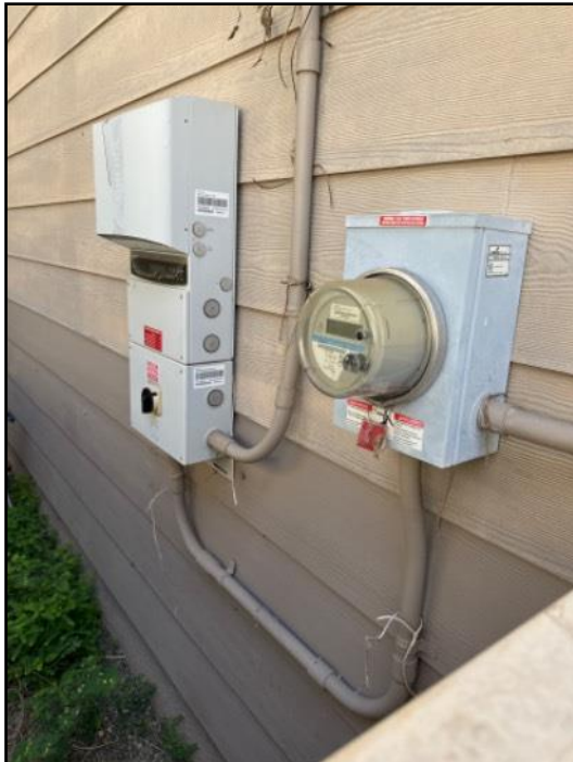
Solar panel meter/monitor
