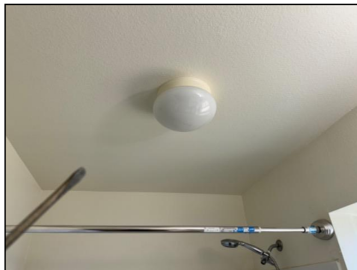
Inoperative @ guest bathroom
