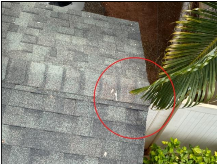
Trees or shrubs too close to building
